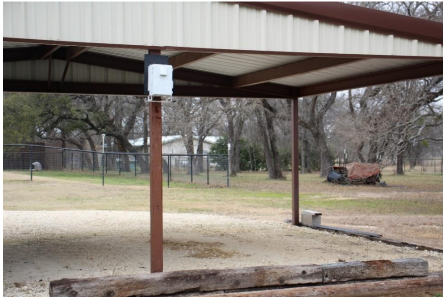
Exhibit 6 Installation of Monitor at Wolf Hollow Site
